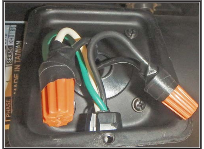
Figure 57. W1873/W1874 motor junction box.
