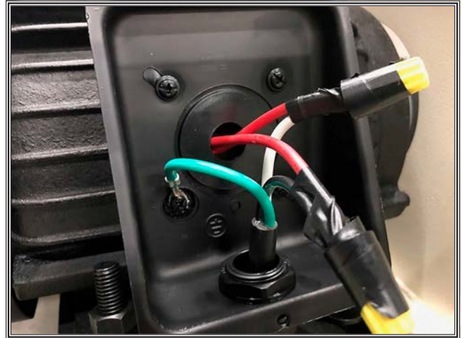
Figure 69. W1865 motor junction box.
