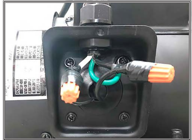
Figure 64. W1863 motor junction box.
