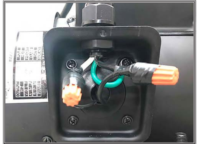
Figure 62. W1862 motor junction box.
