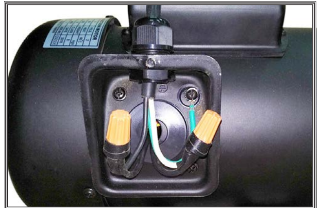
Figure 67. Motor junction box connections.
