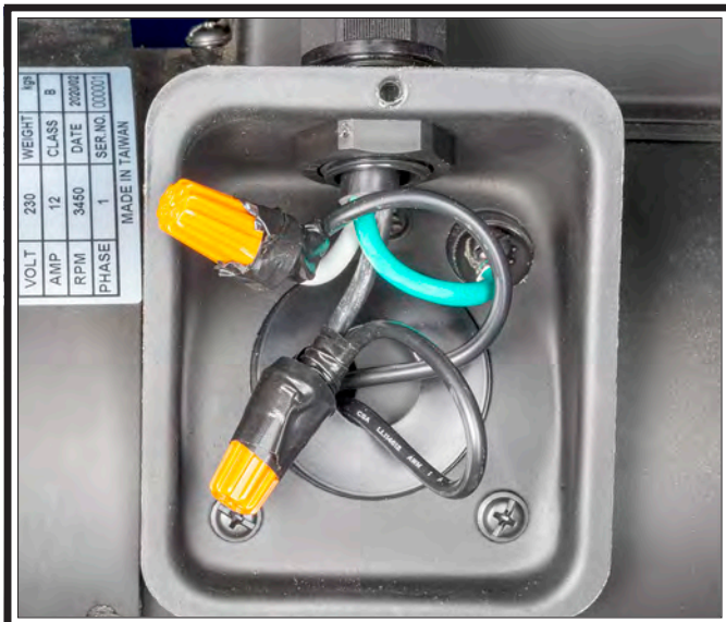
Figure 70. SB1108 motor junction box.
