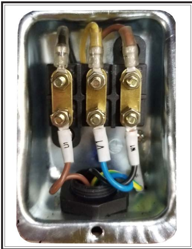
Figure 70. Coolant pump motor wiring (220V) (M1).
