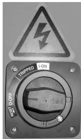
Main power isolation switch
