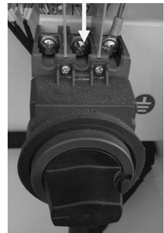
Main power switch
