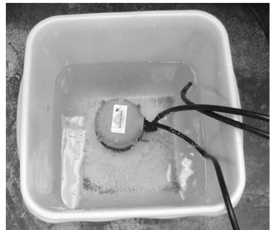
Pump in water container
