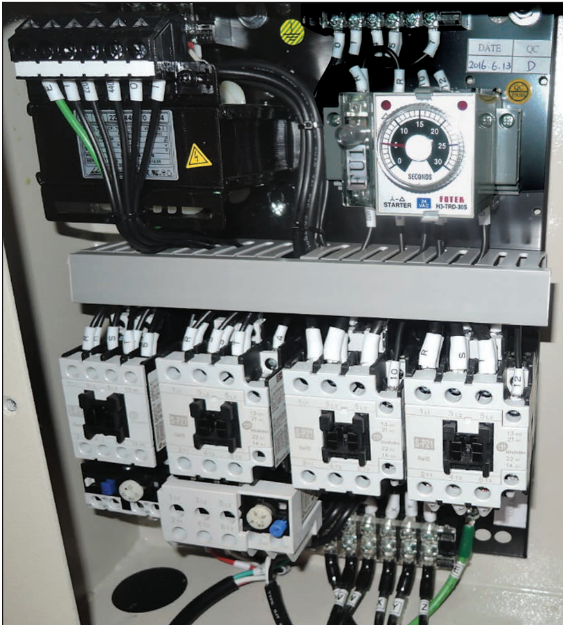
Figure 174. Electrical panel wiring.
