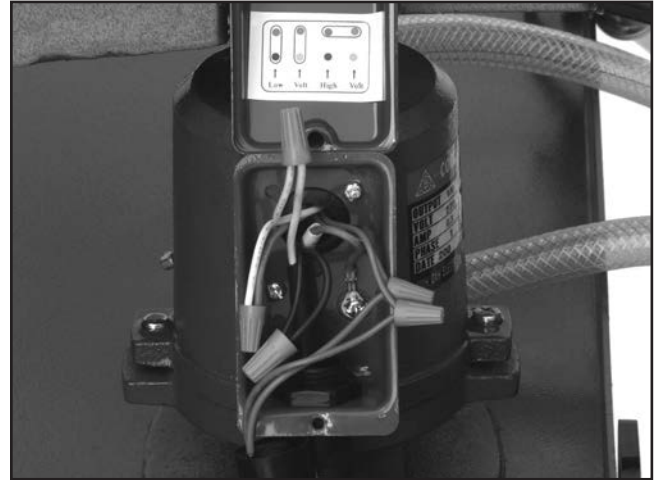
Figure 50. Pump motor wiring.
