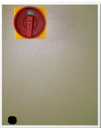
Fig. 3 Electrical Isolating Switch
